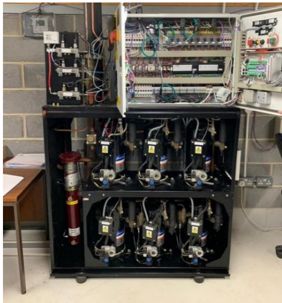
Figure 4: Compressor pack and controller used at the Riseholme Refrigeration Research Centre.
