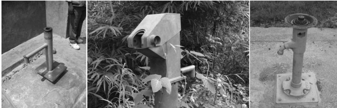
Fig. 1 Broken water infrastructure in Sub-Saharan Africa
